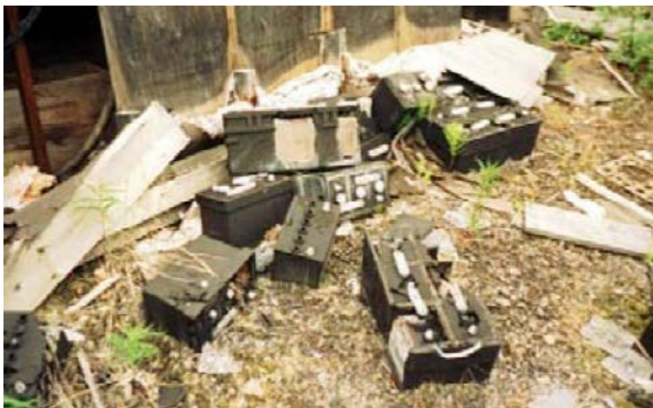
Improper Outdoor Storage of SLABs
